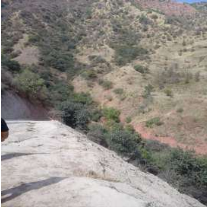
Figure 10 – Existing road at km 9.3 with serious safety deficiencies
